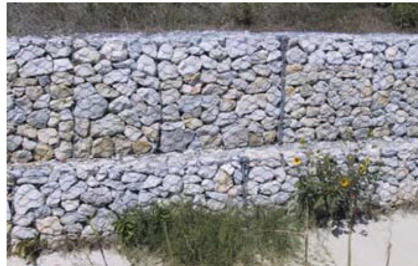
Figure 24: Photograph of rock gabion wall. NRCS 2007b.
